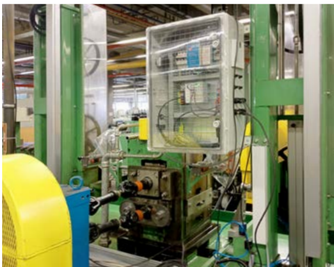
This control center collects data from sensors on the production line at Trützschler
